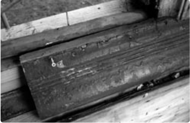
THERE WERE LAYERS AND LAYERS OF LEAD PAINT ON LVPC'S EXTERIOR TRIM. IT WAS CAREFULLY REMOVED BY A LEAD ABATEMENT CONTRACTOR.
